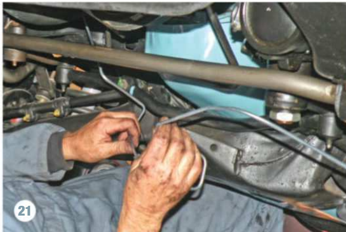
21 We found that the toughest part of the job was running the front line from the distribution block across the crossmember, under the engine, and over to the passenger-side wheel cylinder. The line hangs behind the crossmember and is protected there from ground contact and road debris.
